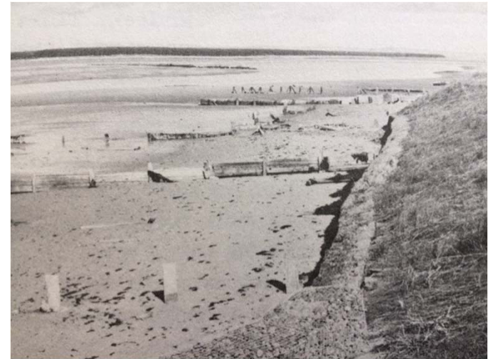
Reproduction of photograph of the coastal defences along the south side of the Eden estuary, 1979. Photograph from Ritchie (1979).
