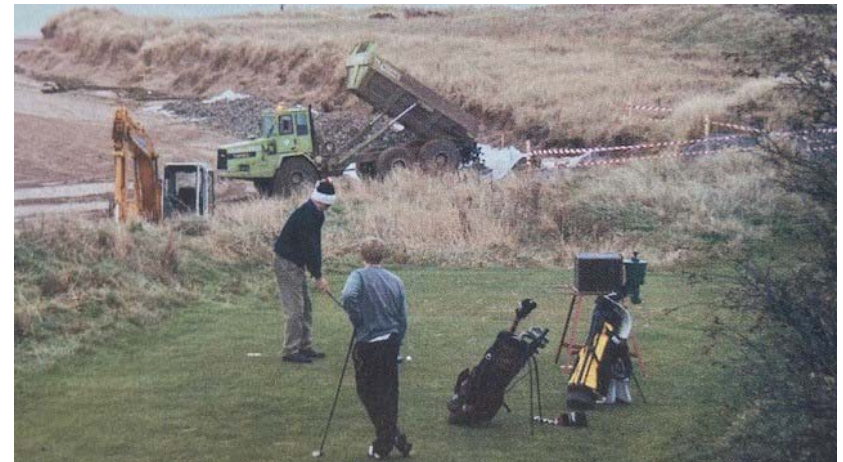
Sediment recharge adjacent to 8th tee of Jubilee golf course, 2008. Photo courtesy of Gordon Moir.
