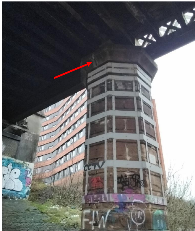
Photograph 4: Example of potential roost feature on pier (red arrow)
