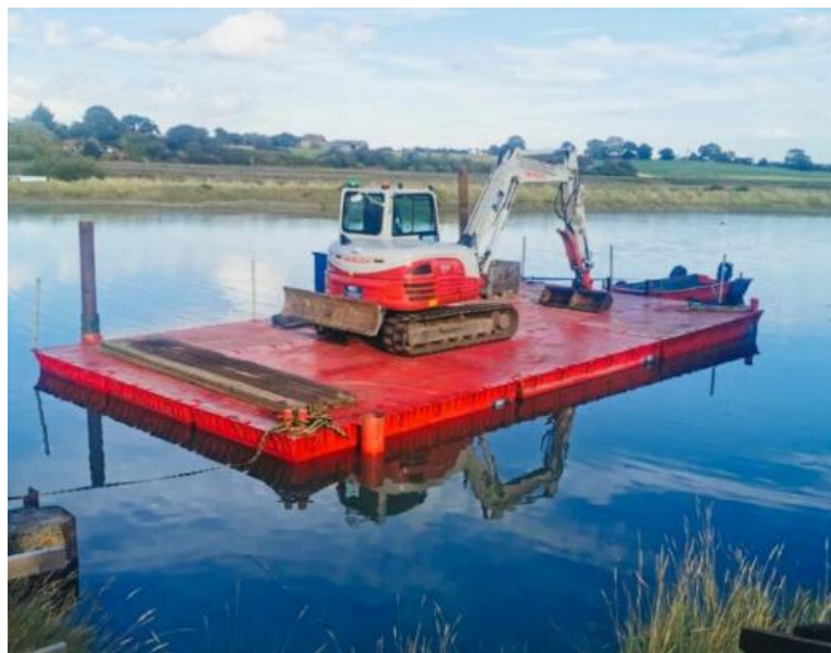
Figure 29 - Example of Floating Pontoon
