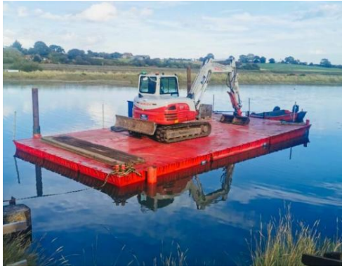
Figure 35 - Example of Floating Pontoon
