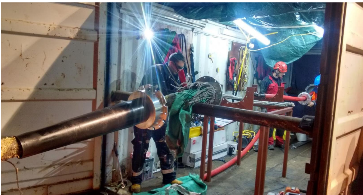
Figure 14. Orbital Marine Power and HV Contractors offshore on a multi-cat vessel cable jointing or “splicing” operations where static cables are permanently connected to the platform cable which supplies power and communications.
