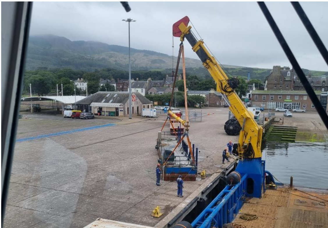
Figure 2 – Pontoon Lifting Arrangement (KOF pictured carrying out the lift however the slinging arrangement will remain the same)
