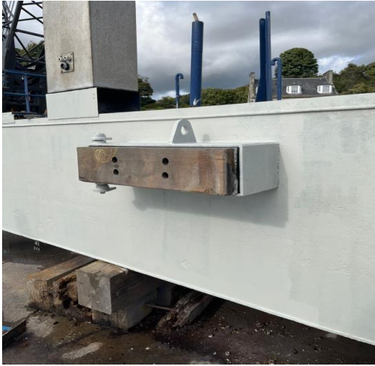
Fig-5 Old fendering to be replaced with new.
