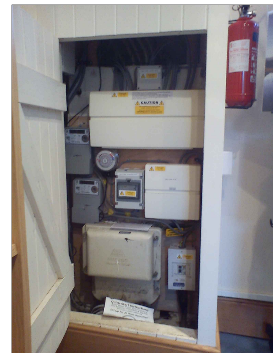
Photo 1: Existing electrical board inside visitor center for connection to provide power for NG treatment plant and UVC-032 Chamber
