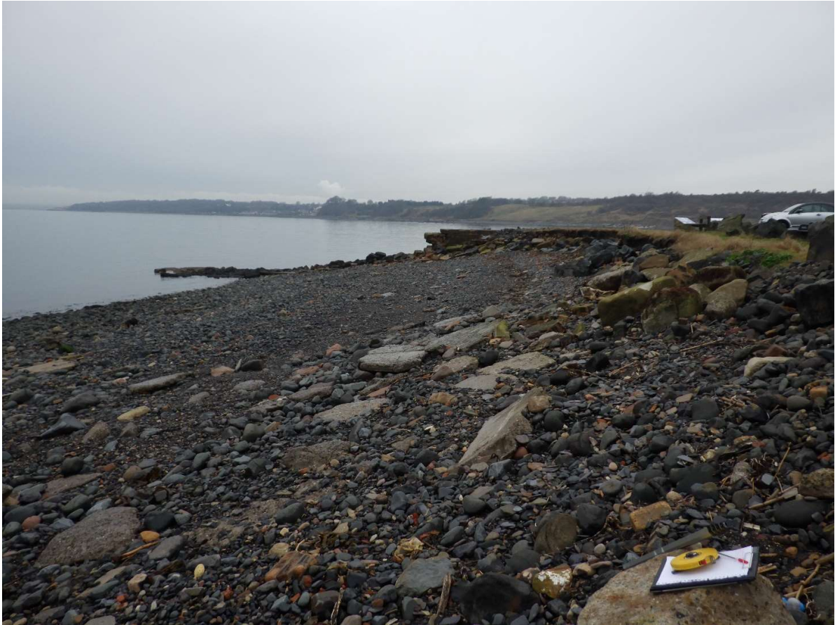
General View of the Eroding Section of Coast Looking in an Westerly Direction
