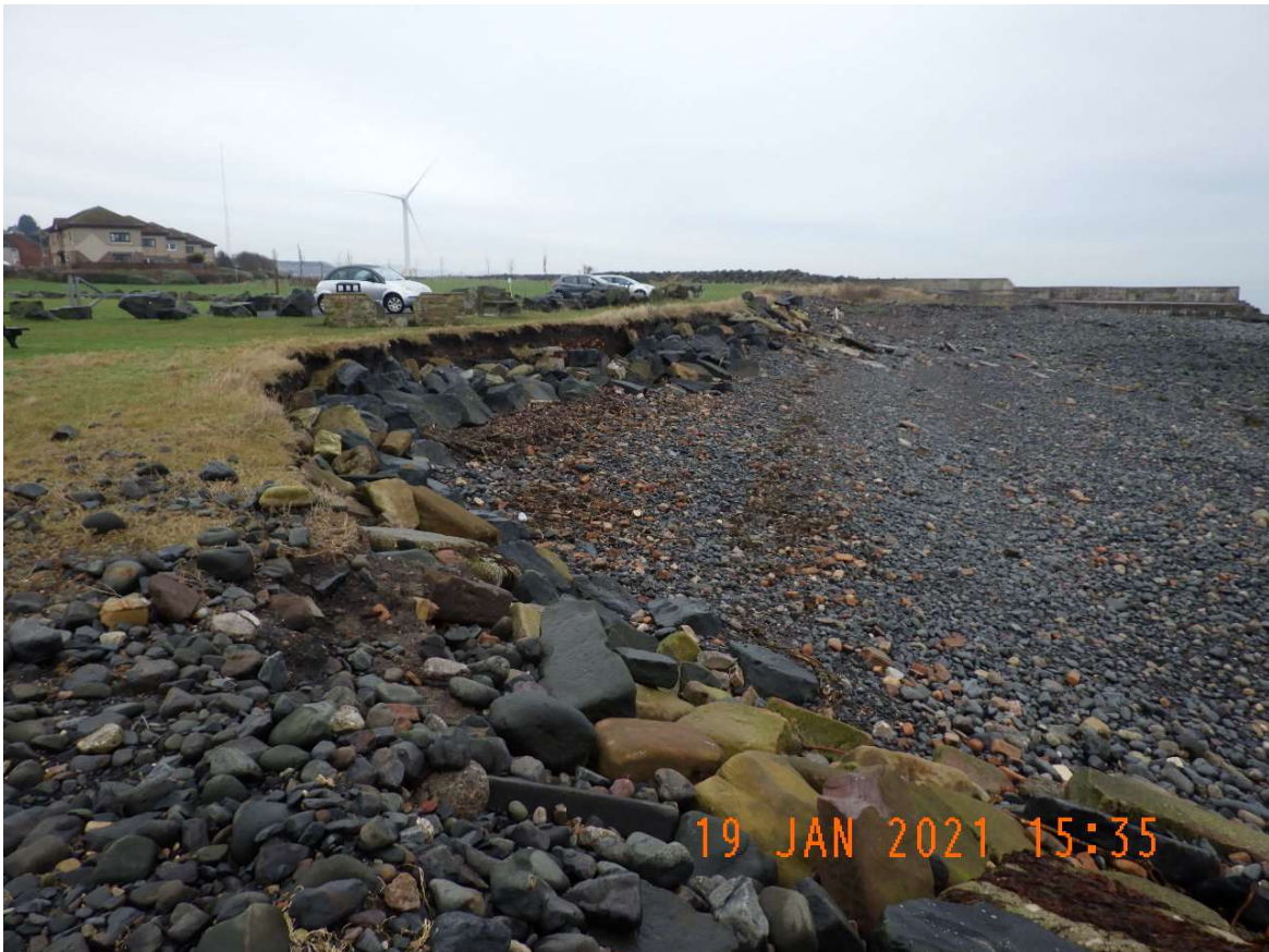
General View of the Eroding Section of Coast Looking in an Easterly Direction
