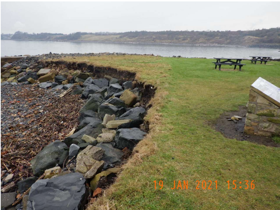
General View of the Eroding Section of Coast Looking in an Westerly Direction Showing the Proximity to the Historical Information Sign and Picnic Area
