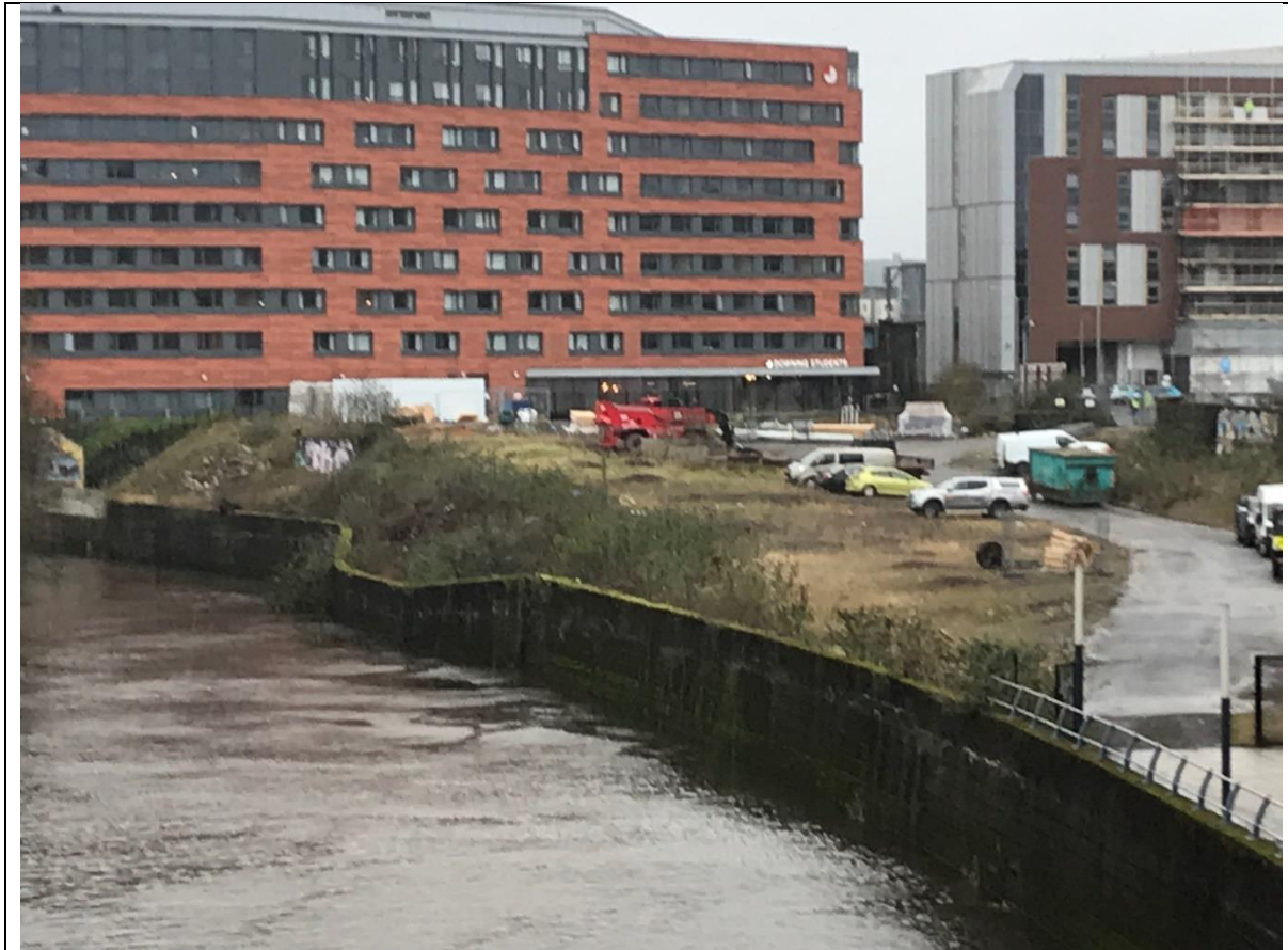
Site Looking West , highlighting section of partially collapsed quay wall
