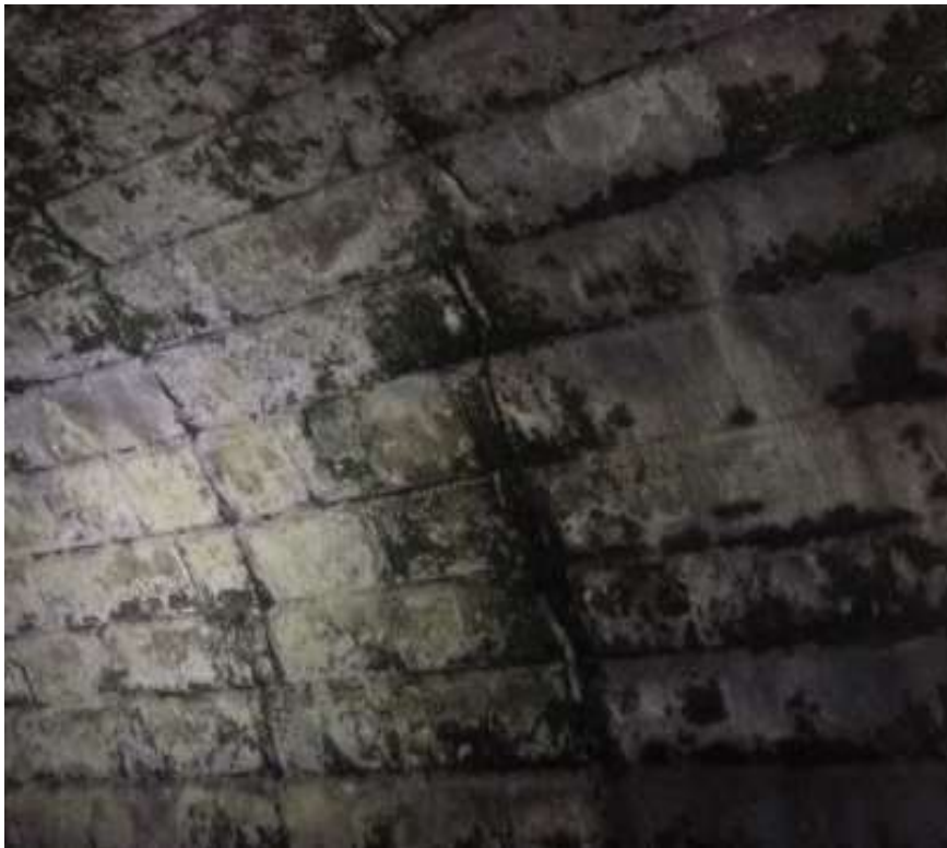
Cracks within structure
