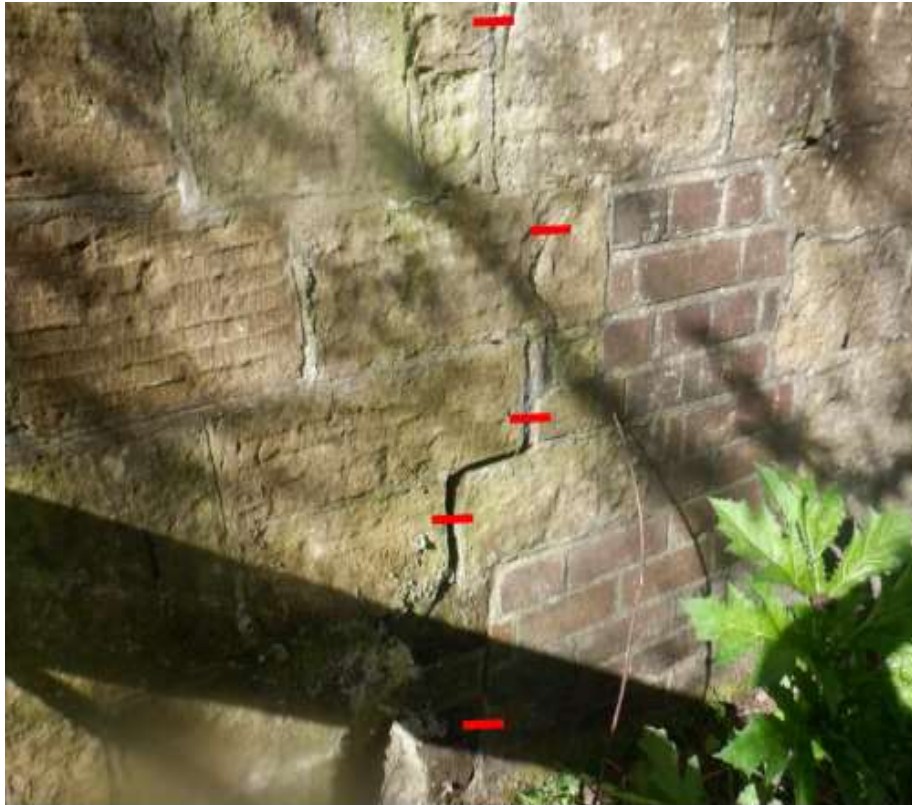
Example of cracks
