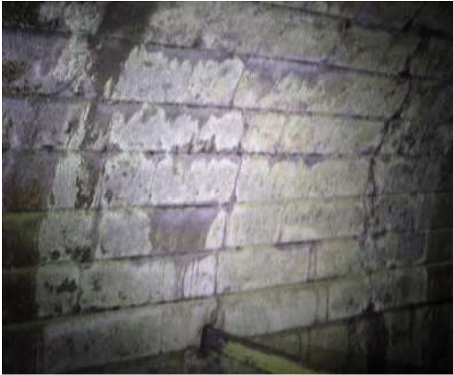
Cracks within structure
