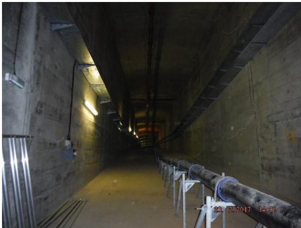
Figure 5, A87 Skye Bridge – Typical internal view from within the box girder, showing the water main and cable trays.
