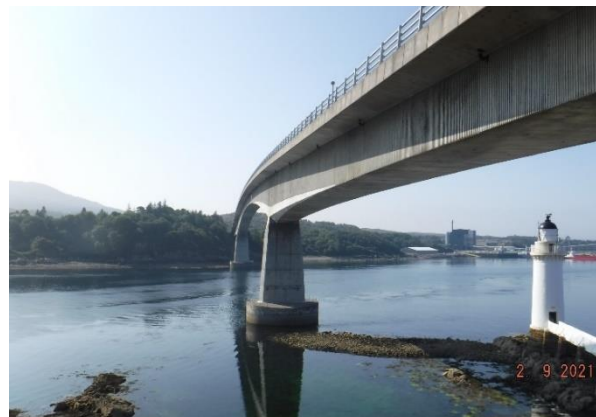
Figure 8, A87 Skye Bridge – Typical view of the bridge piers, concrete box girder and parapet from below the bridge.
