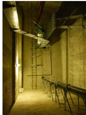
Figure 6, A87 Skye Bridge – Typical internal view from within the box girder at one of the main piers, showing the water main, access ladder, drainage and cable trays.
