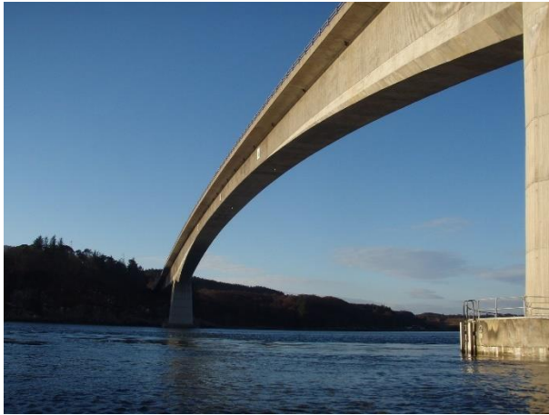
Figure 3, A87 Skye Bridge – Typical view of the bridge box girder across the tidal channel (span 4)
