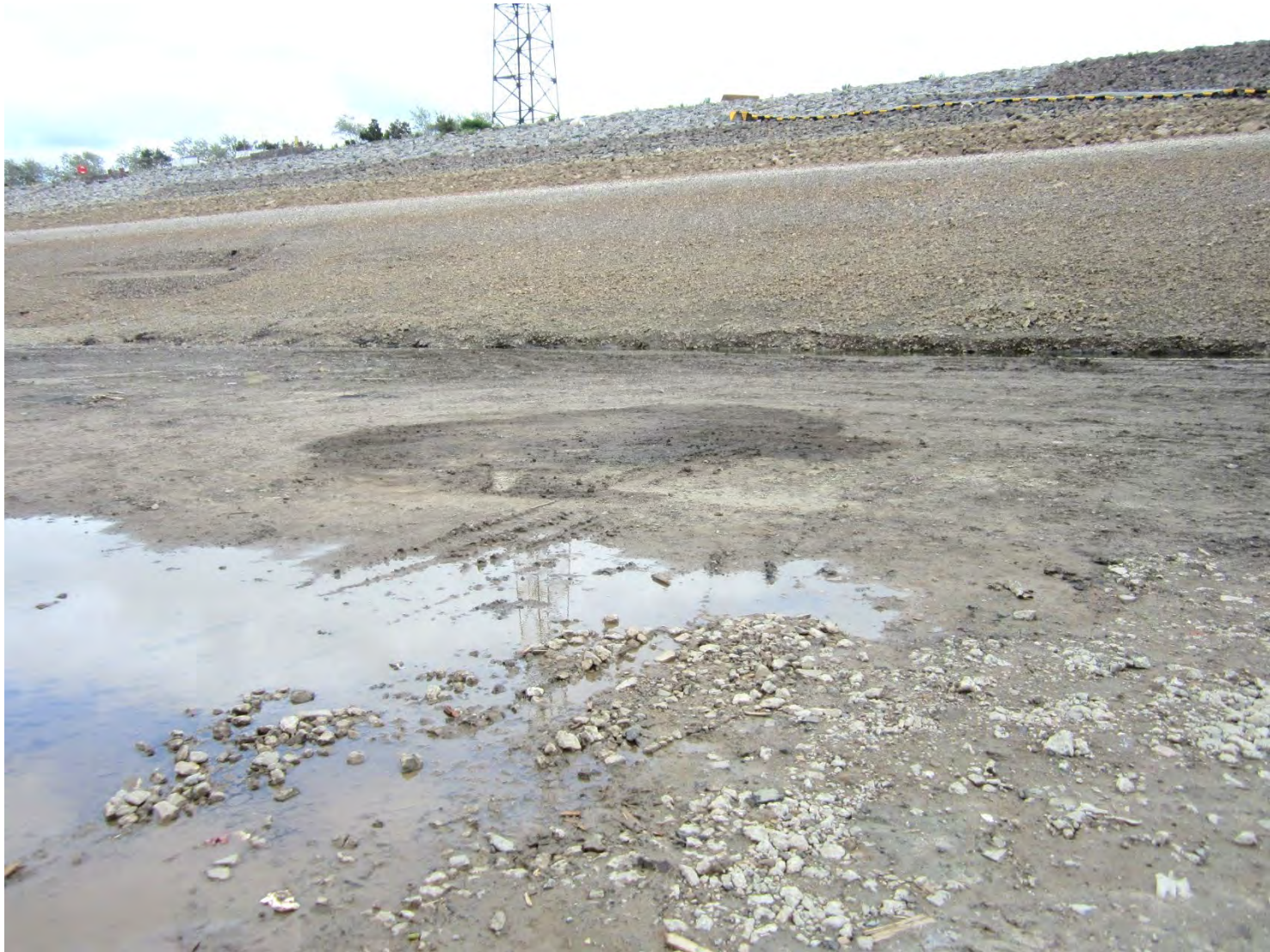
view from middle of the inner dock when 'dry' towards the East and proposed berthing quay
