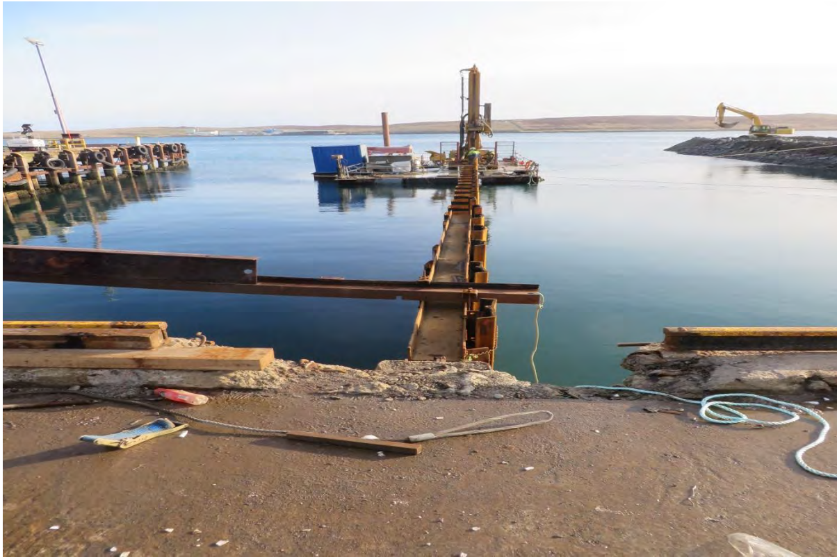
Drilling rig for pre-treating hard strata on pile clutch line ahead of piling
