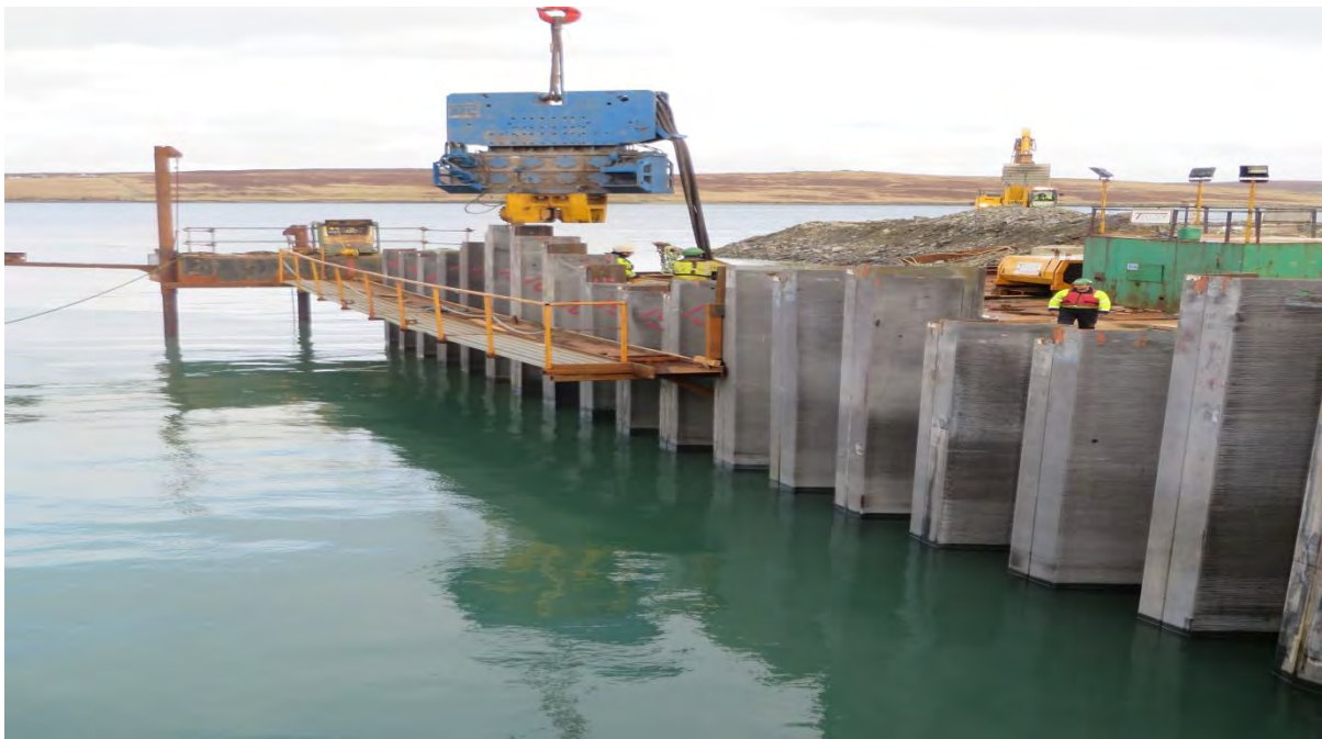
Vibro hammer piles to final level level in to blasted pre-treated trench
