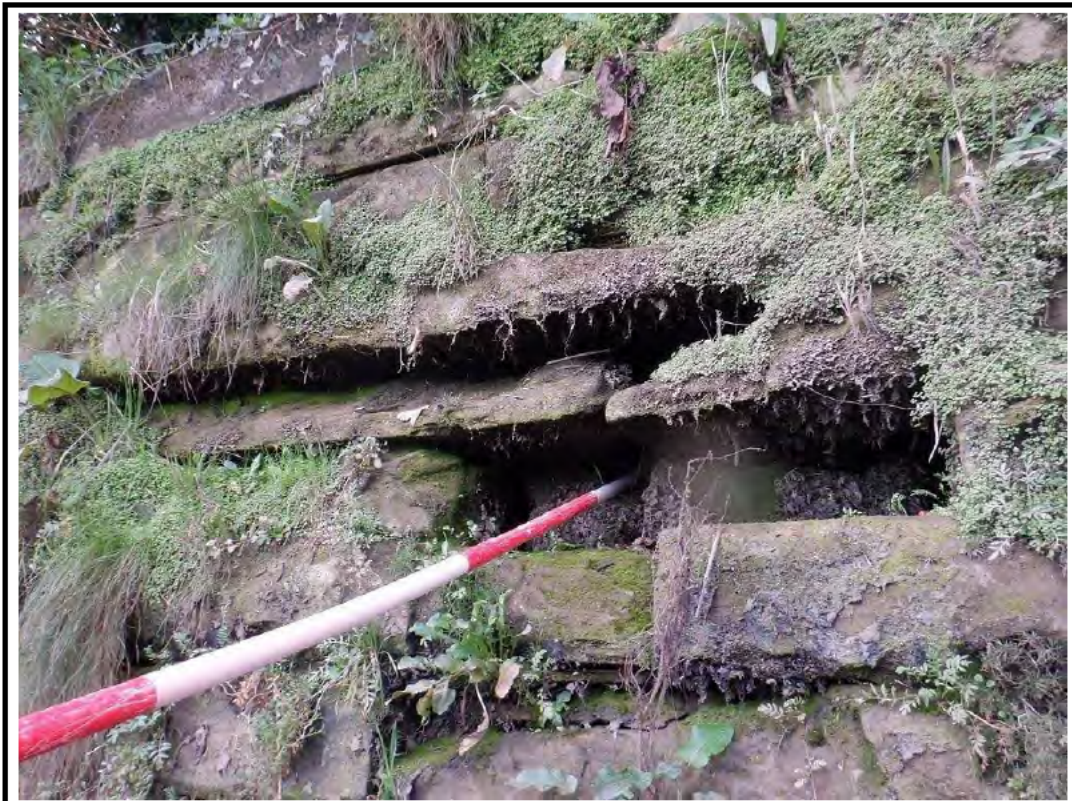
PHOTO 14: P14 - AREAS OF VOIDING AND SPALLING LOCATED THROUGHOUT 14/09/20
