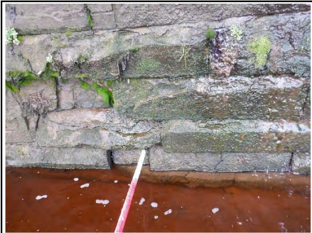
PHOTO 18: P18 - AT 9M FROM THE ABUTMENT SPALLING AT WATER LEVEL, 14/09/20
