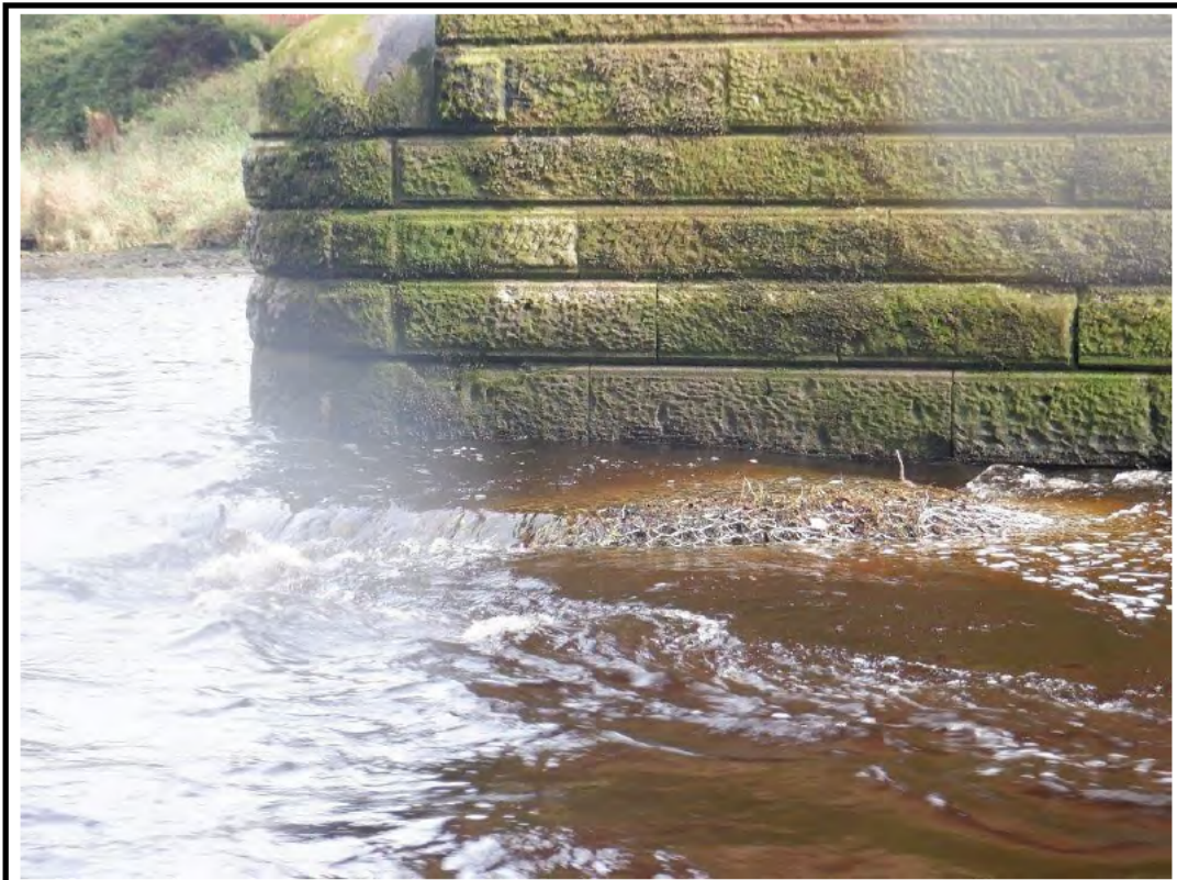
PHOTO 6: P6- PIER 3 DAMAGED GABIONS 14/09/20
