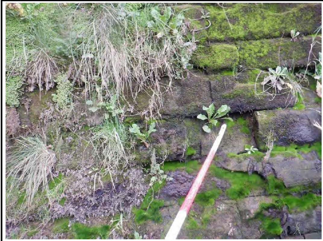
PHOTO 17: P17 - 8M FROM THE ABUTMENT 4M2 SPALLING 14/09/20
