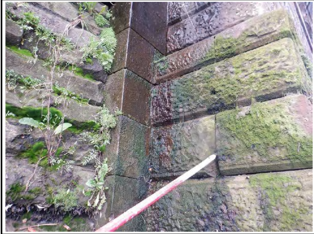
PHOTO 21: P21 - DOWNSTREAM RETURN - FRACTURE 14/09/20
