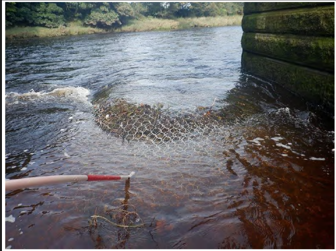
PHOTO 7: P7- PIER 3 DAMAGED GABIONS 14/09/20
