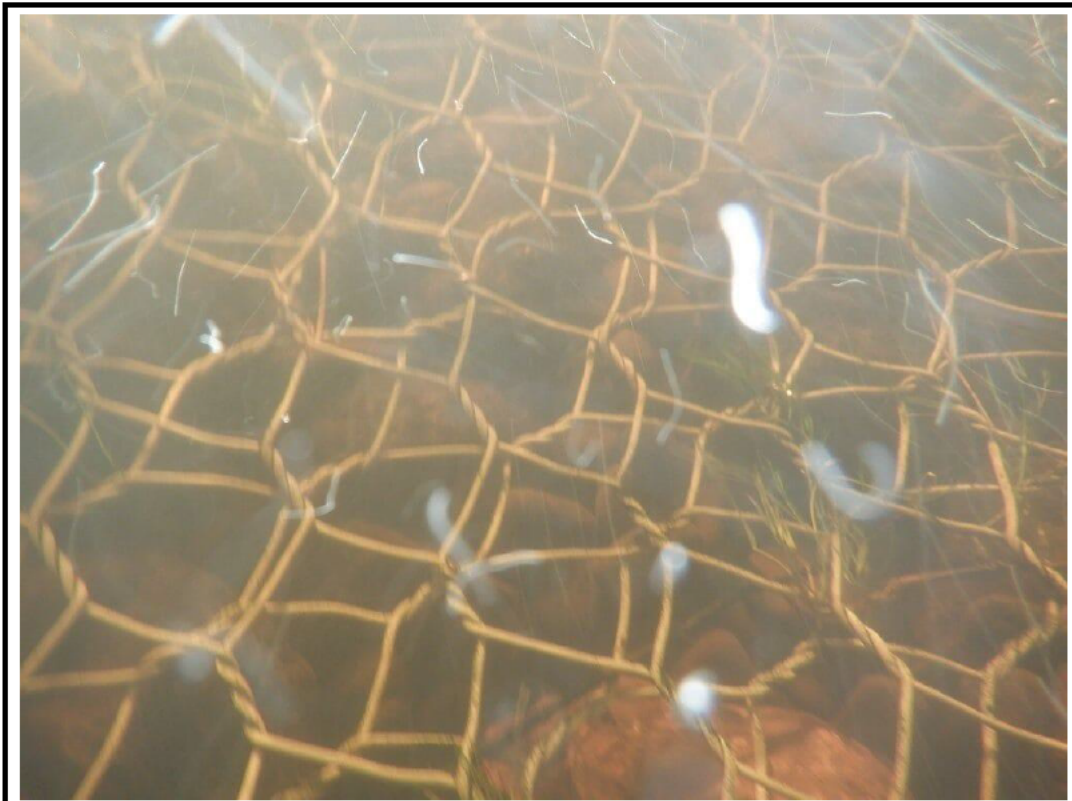
PHOTO 10: P10- PIER 3 DAMAGED GABIONS 14/09/20
