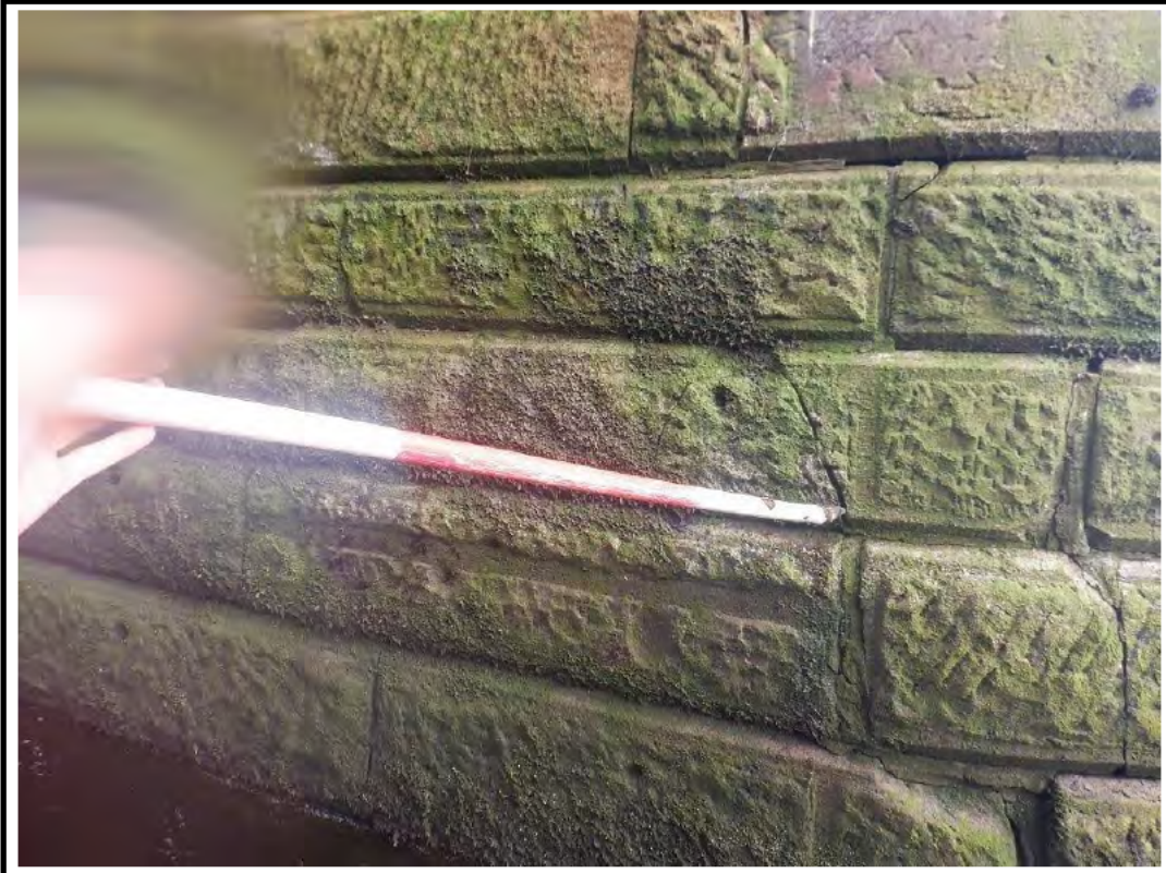
PHOTO 29: P29 - 2NO VERTICAL FRACTURES 14/09/20
