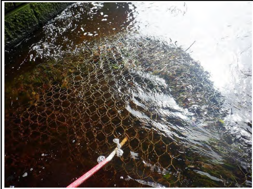
PHOTO 9: P9- PIER 3 DAMAGED GABIONS 14/09/20
