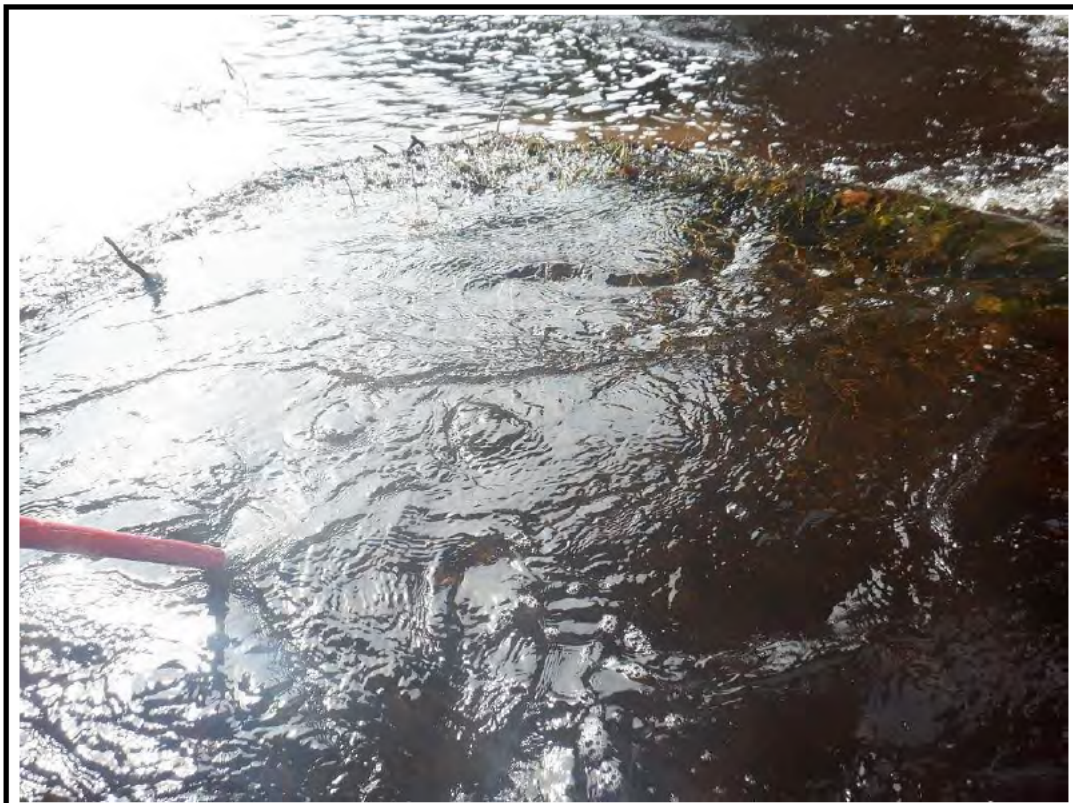
PHOTO 8: P8- PIER 3 DAMAGED GABIONS 14/09/20
